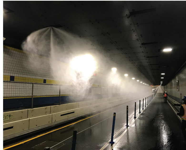
Testing of fixed fire suppression system in Hugh Carey Tunnel
