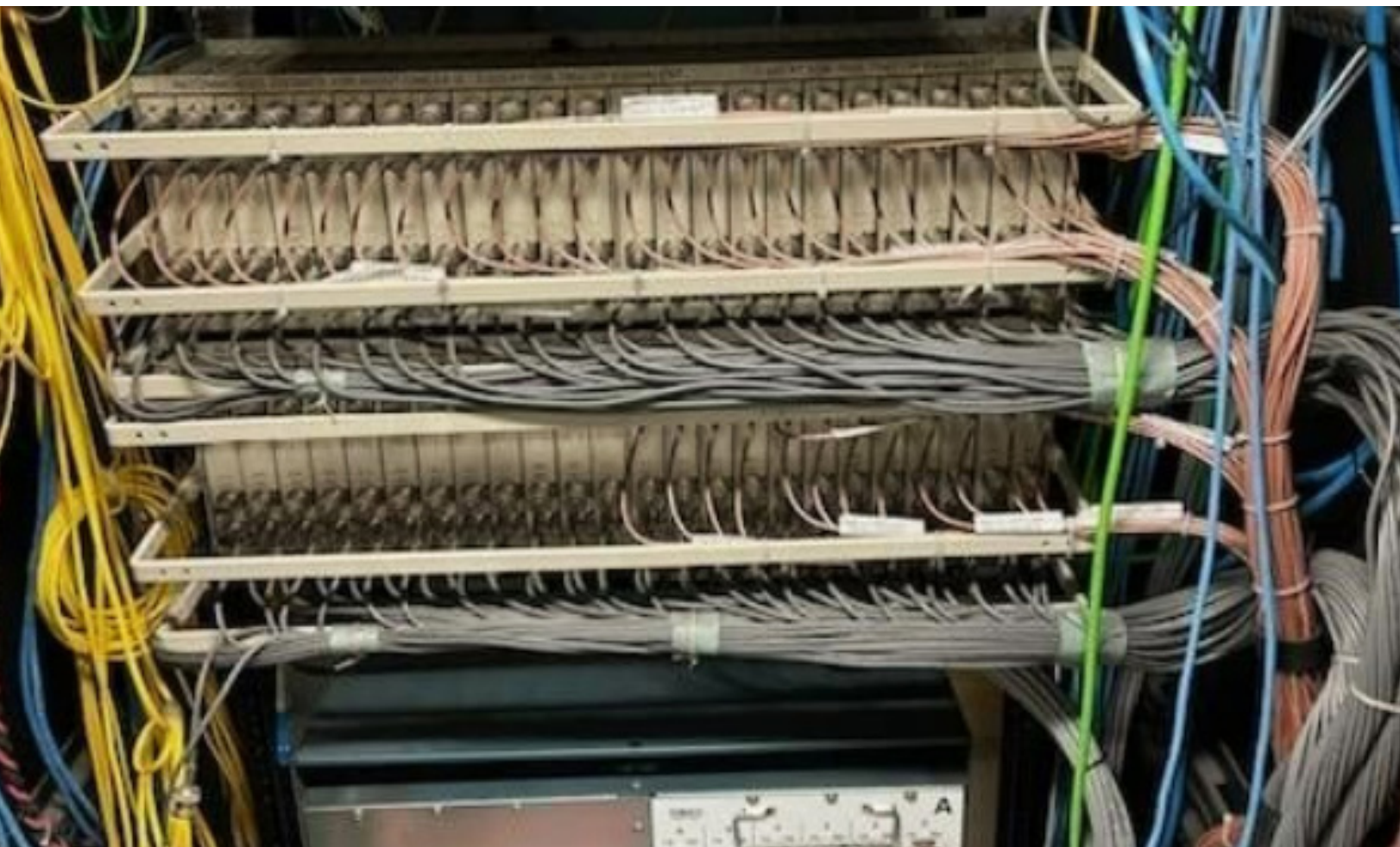
Metro-North's SONET communications systems equipment
