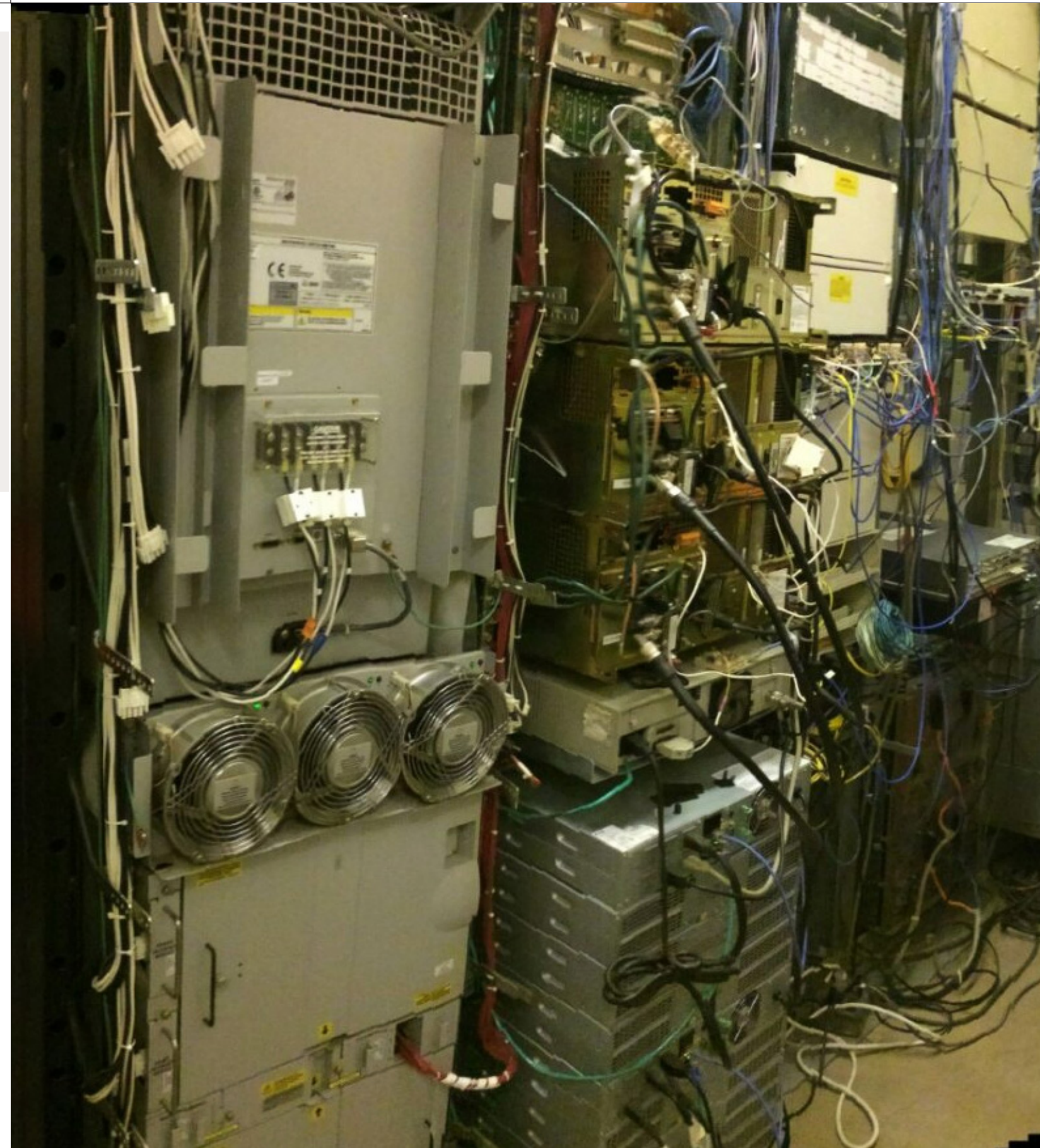
Communications room interior
