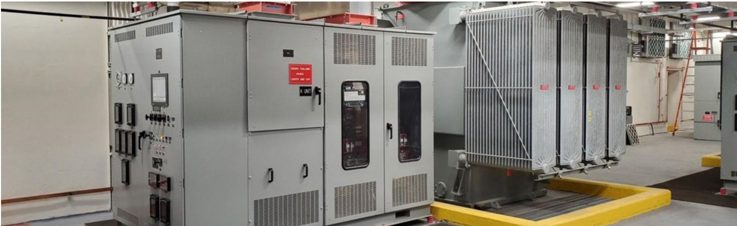
Maspeth Substation, NYCT
