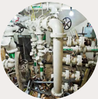
Pump rooms (ROW)
