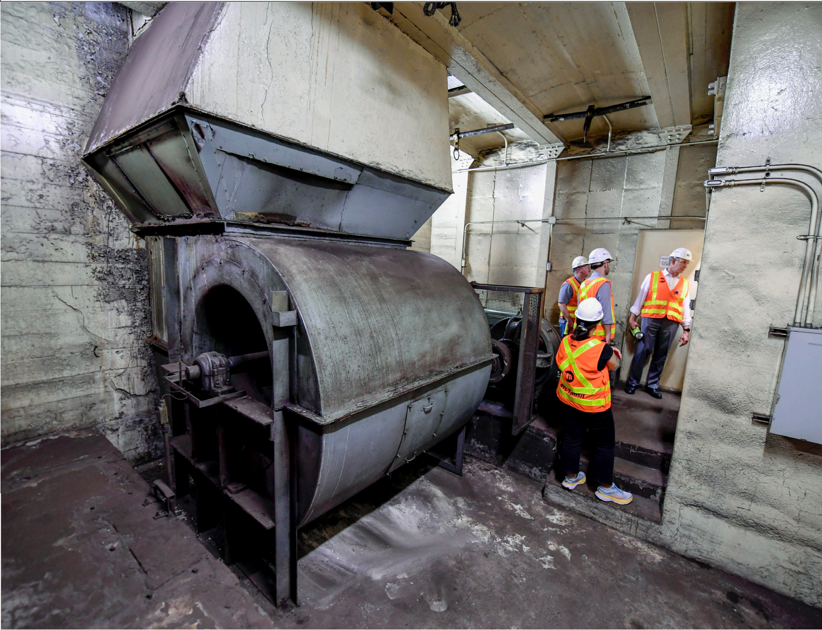
Prince Street Fan Plant
