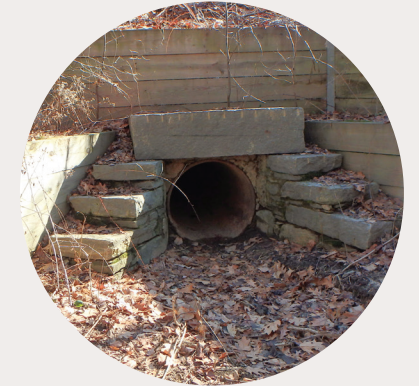
Culverts Are designed to allow water to flow underneath tracks to manage drainage and prevent flooding.
