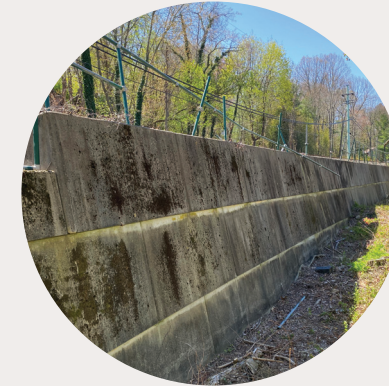
Retaining walls Built to hold back soil and provide support for our elevated structures or keep steeply sloped surfaces from collapsing onto the adjacent track bed.
