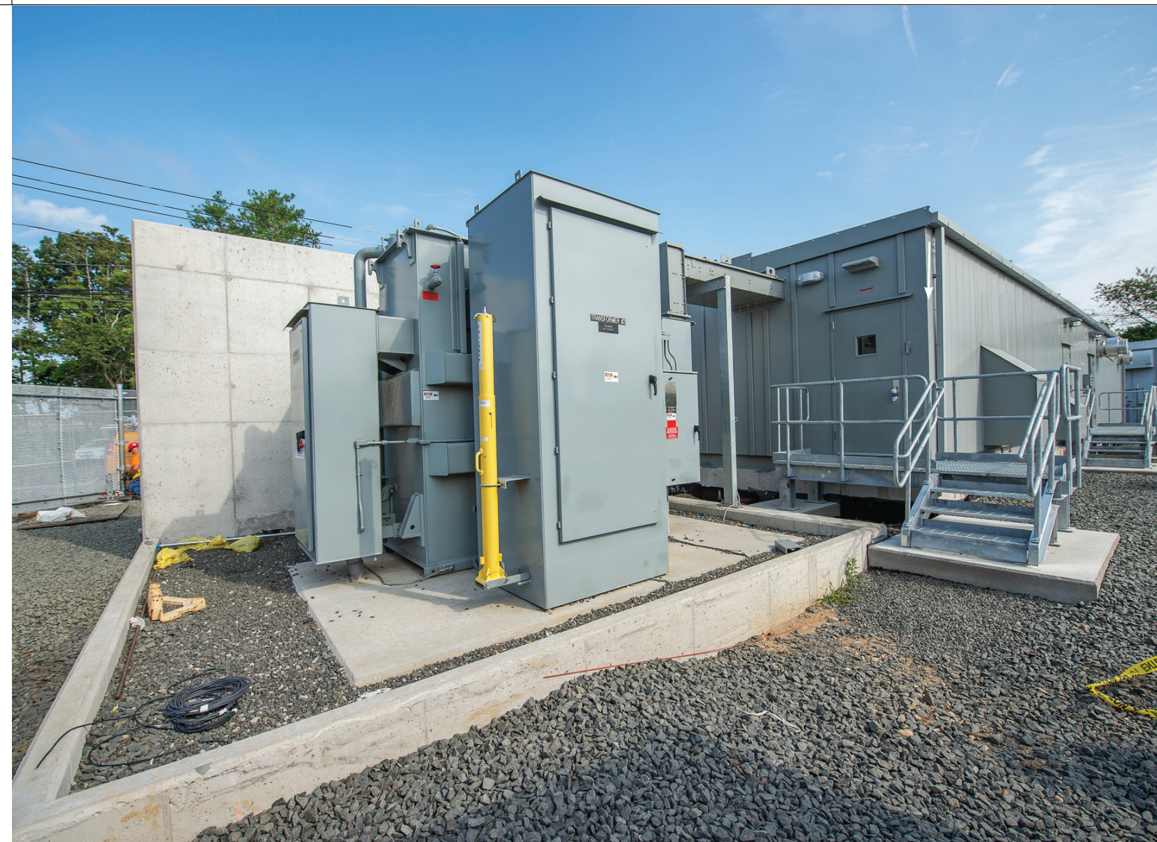
Left page, third rail. Above, New Cassel Substation
