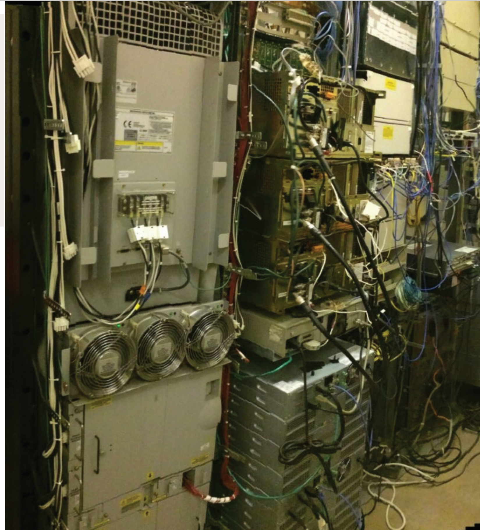
Communications room interior
