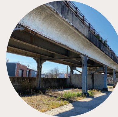
Viaducts Provide separation of the railroad from the surrounding community or allow our rail system to traverse a wide valley with a bridge-like structure.
