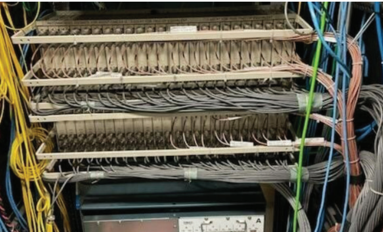
Metro-North’s SONET communications systems equipment
