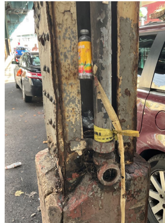
Rusted steel structure
