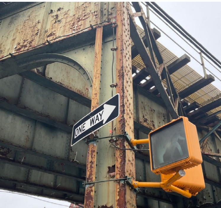
Rust and deterioration on the West End Elevated
